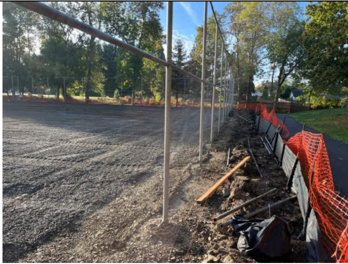
Figure 3 Existing 10' tall fence posts – re-set by contractor into alignment.
